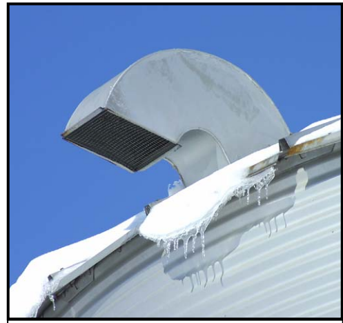
Photo 2 -- Roof vent with horizontal opening, which allows blown-in snow.
